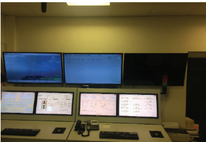
Der Control-Room des Engine-Room-Simulators 1/2
